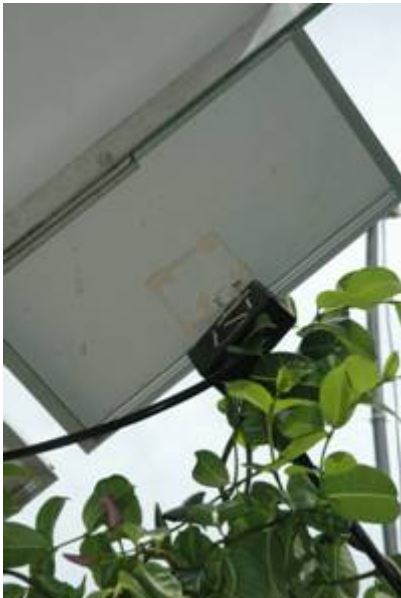
Figure 1 Junction box pulled off the base of the panel from the weight of the creeper vines
